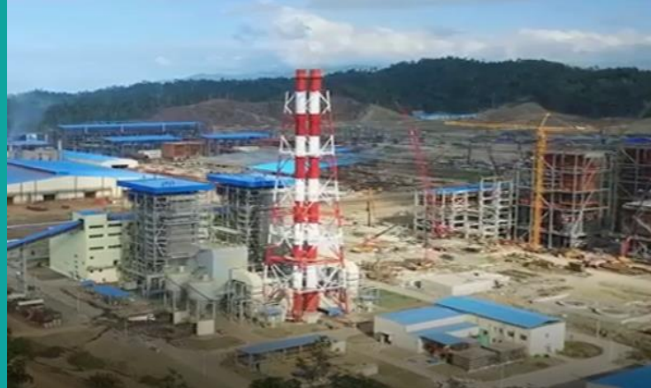
1.26GW Coal Fired Power Station
