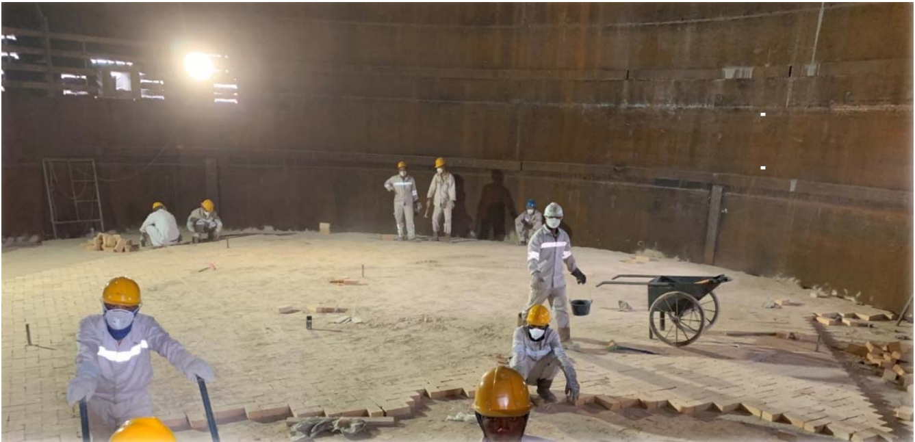
Refractory lining of Hengjaya Nickel's electric furnace
