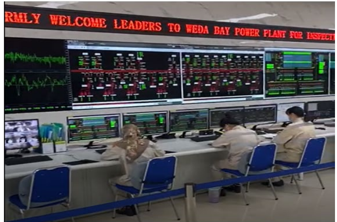
Weda Bay Power Plant control room
