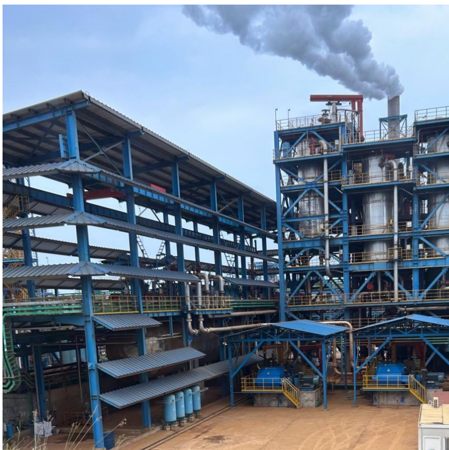
View of HNC operations
