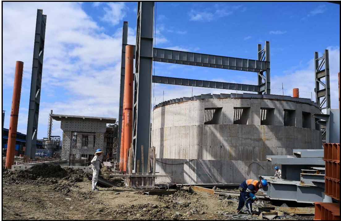
Base of electric furnace.
